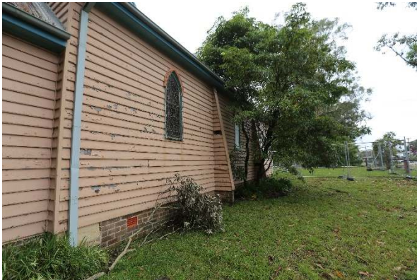
Figure 46. Flaking paint and damaged cladding to southern elevation.
