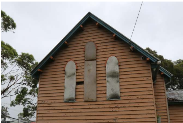
Figure 44. Damaged cladding to eastern elevation.
