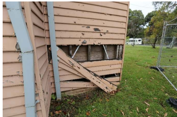
Figure 45. Damage to cladding at south-eastern corner.
