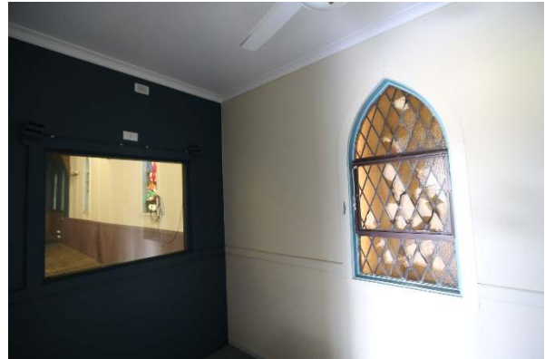
Figure 47. Porch. Broken glazing visible in window.
