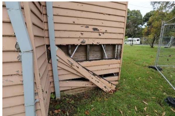
Figure 45. Damage to cladding at south-eastern corner.
