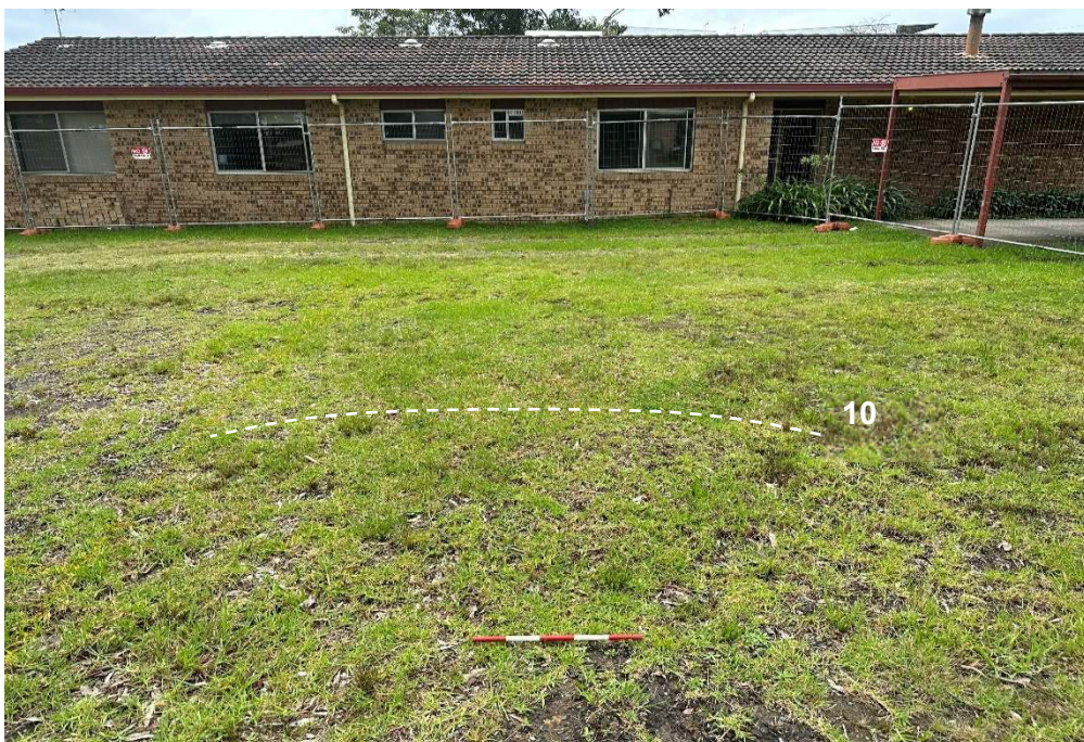
Figure 61. Examples of micro-rises of the ground surface (white dashed line) (width shown) in the northern portion of Lot 7, facing north.
